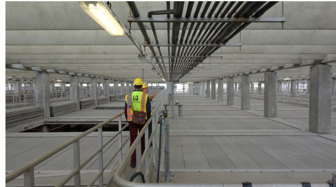
— Westpoint Treatment Plant
