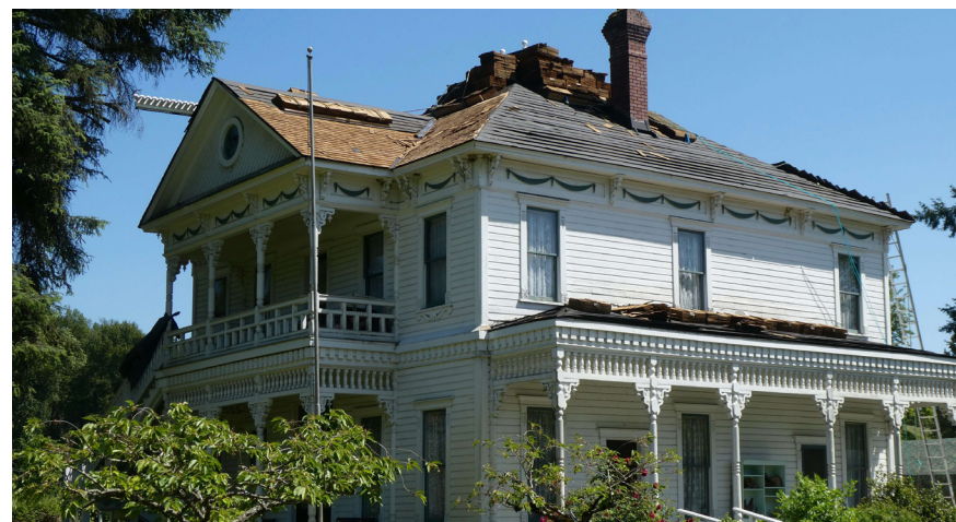
In the process of tearing off old shingles and installing new, cedar shingles, original skipjack boards were exposed on the east side of the Neely Mansion roof, 2023. Photo: Neely Mansion Association, Linda Van Nest
